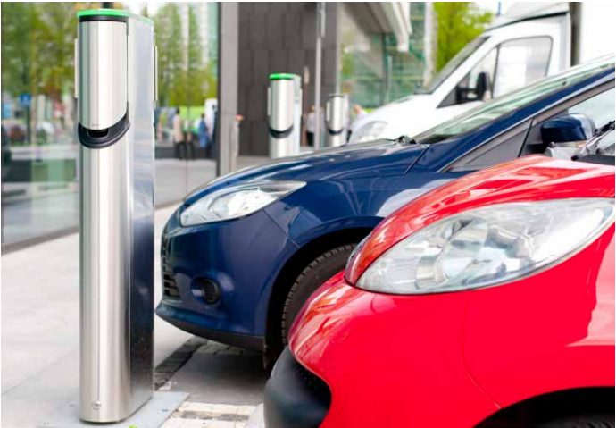
Charging station at Eurocentrum, Warsaw, Poland
