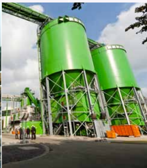
Max Green - Rodenhuize plant - Ghent
