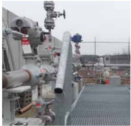
NMP - Ethylene pipeline Antwerp - Feluy
