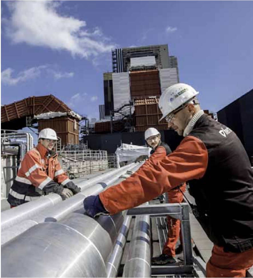
Hertel at Electrabel (Rotterdam)
