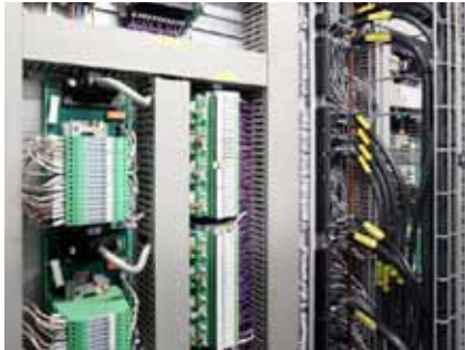
Multitechnics - General and industrial electricity
