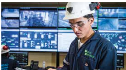
Inside the control room for the Disseminated Ore Body
