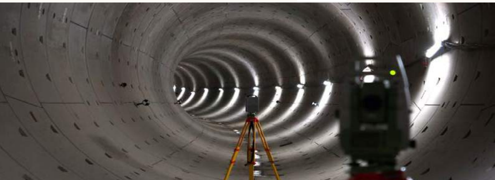
3D Laser scanning of new North/South metro line in Amsterdam, The Netherlands
