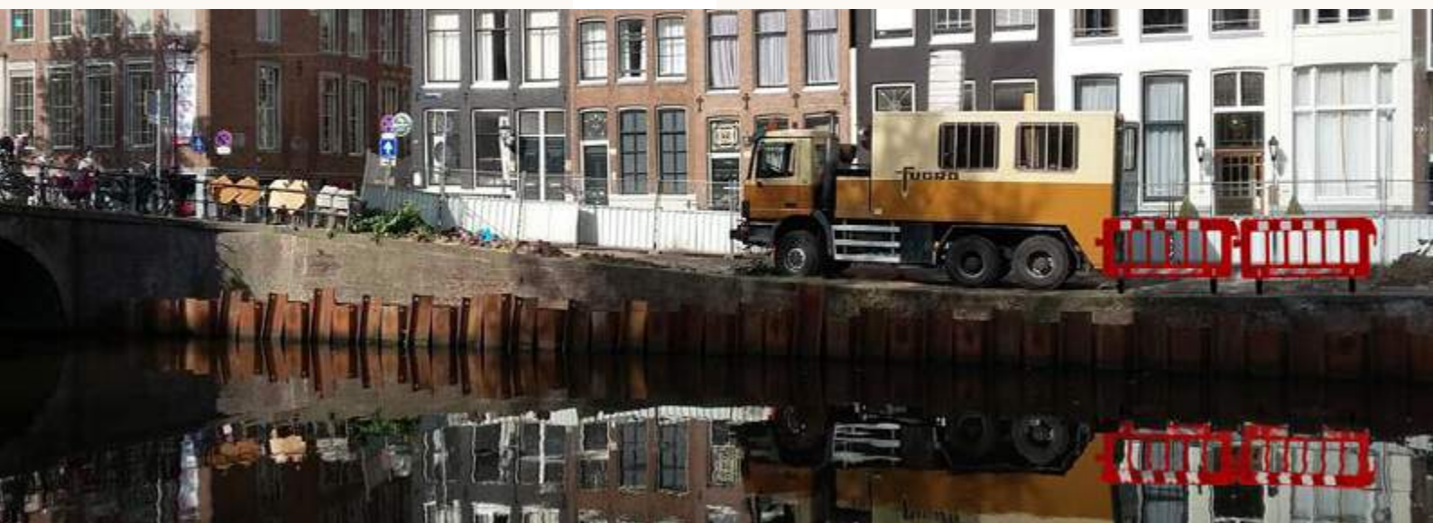
Performing cone penetration tests for reconstruction of quay wall in center of Amsterdam, The Netherlands.
