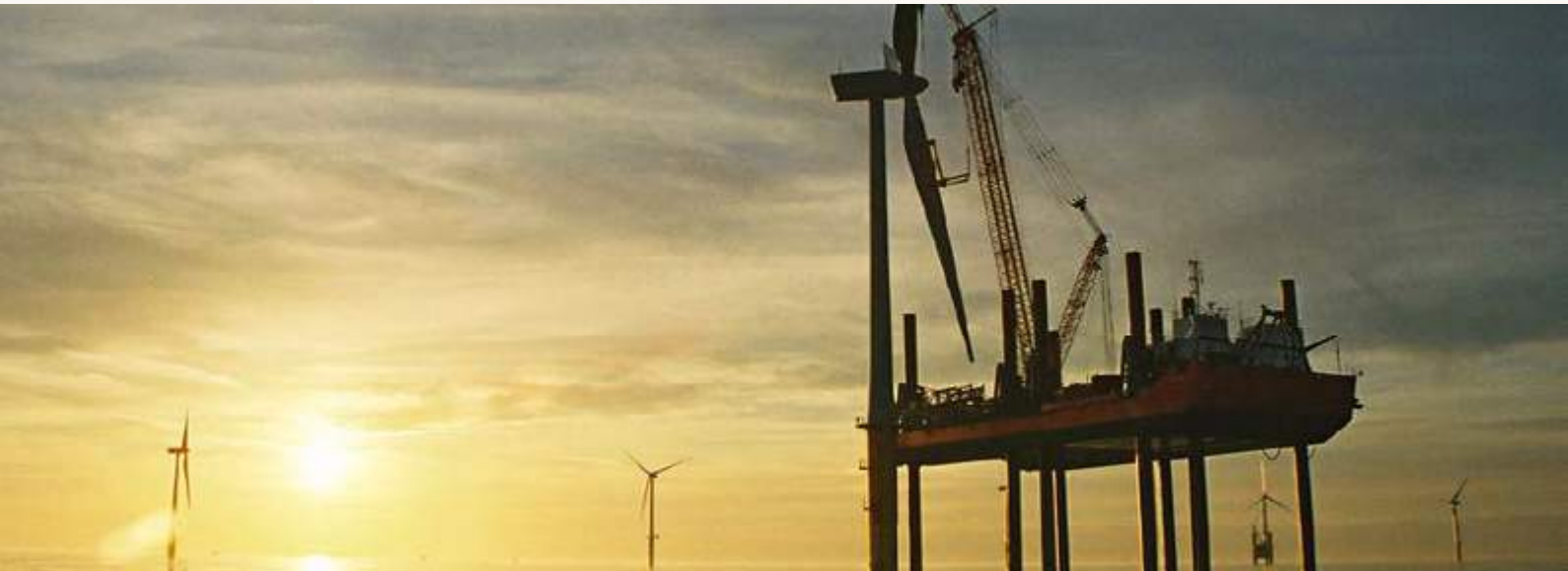
Installation of wind farm project off the north coast of Wales, United Kingdom.
