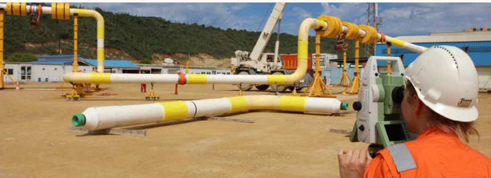
Dimensional control of the spools for deepsea offshore project, Porto Amboim, Angola.
