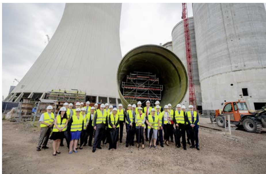
Inauguration of the shell of the natural draft tower at the Kozienice power plant in Poland.
