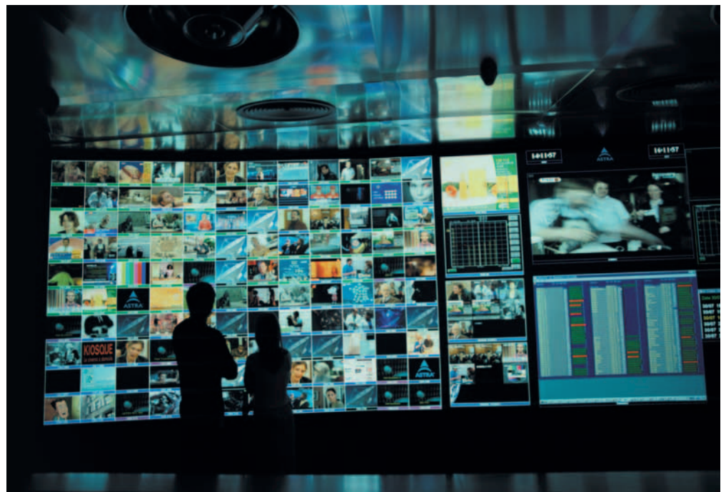
Controlezaal DINO "Digital Network Operation Center"
