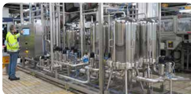
Cold Stabilisation Module (CSM) at the Molson Coors brewery site - Zagreb
