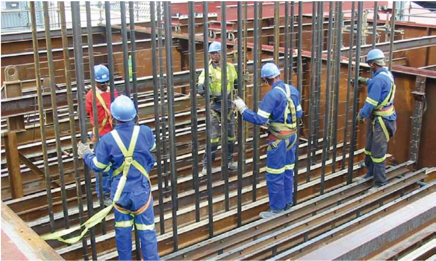
□ Workers installing the electrodes of an ESP in an Eskom power plant, South Africa
