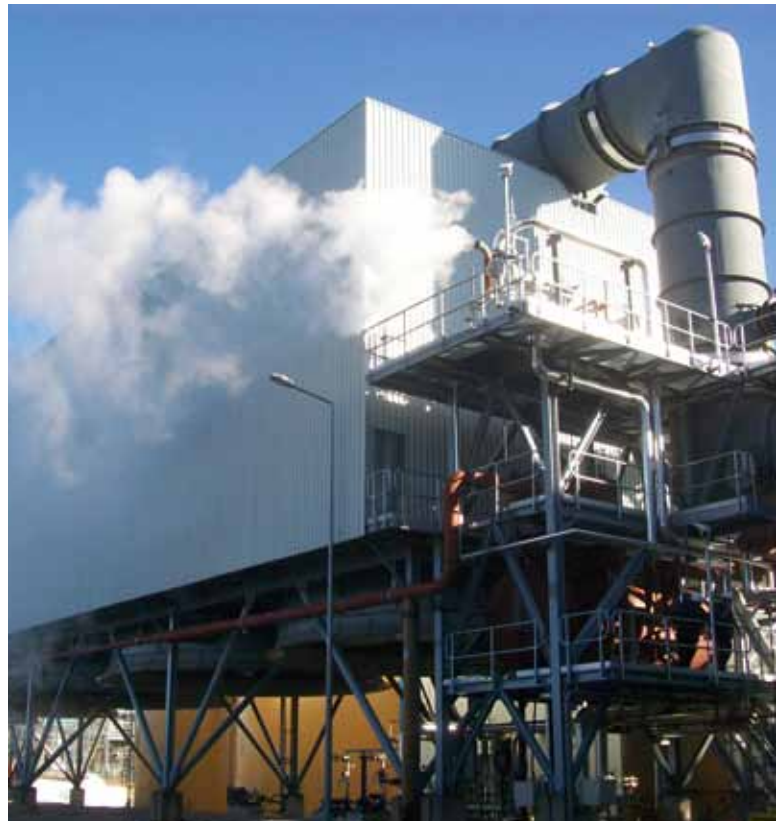
□ Air cooled condenser built by Research-Cottrell in Turkey
