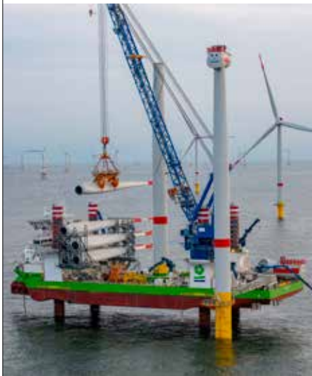
The offshore windfarm Rentel, located in the Belgian North Sea
