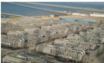
Evaporators in desalination
