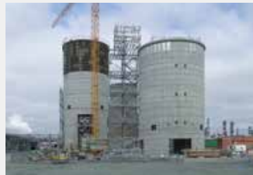
Building and operating of Tricoya® wood chip acetylation plant in Hull
