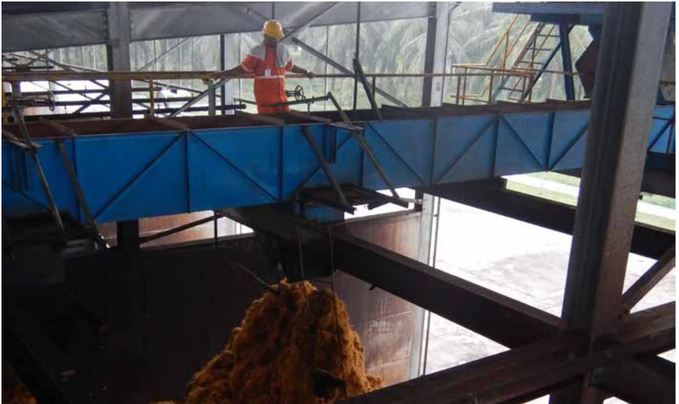
SIPEF - EFB fiber is mixed with waste water in an aerated composting bunker (Bukit Maradja)
