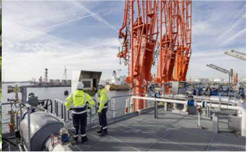
Agidens - Automation of loading arms at Oiltanking Stolthaven Antwerpen
