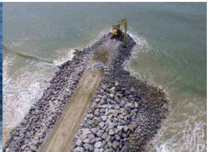
DEME - Construction of a breakwater to protect against rising sea levels in Benin
