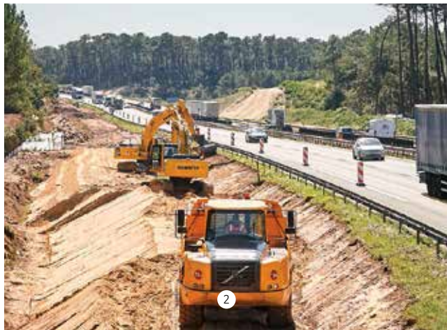
1 The VINCI Autoroutes network comprises almost 4,500 km of motorways in the west and south of France (above, the A11 linking the Paris region to Nantes).
