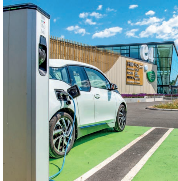
C4's electric car charging points.
