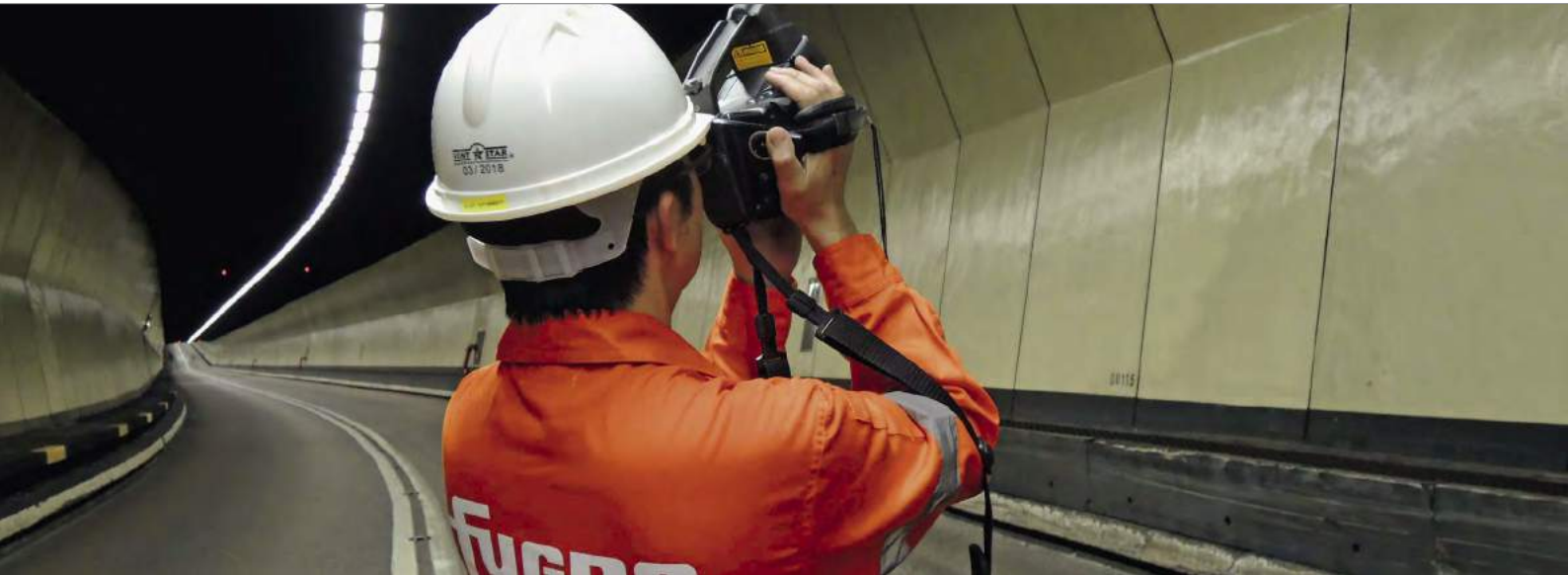
Detecting possible defects in tunnel structure by infrared thermography, Hunghom Cross Harbour Tunnel, Hongkong.
