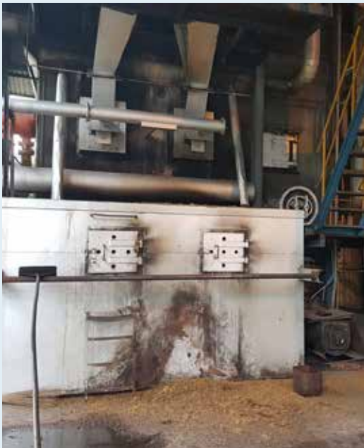
Doors of a boiler furnace
