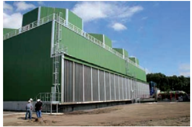
Mechanical draft cooling tower in Germany
