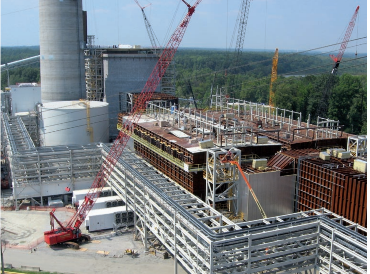
Construction of fabric filters for a power plant in the United States
