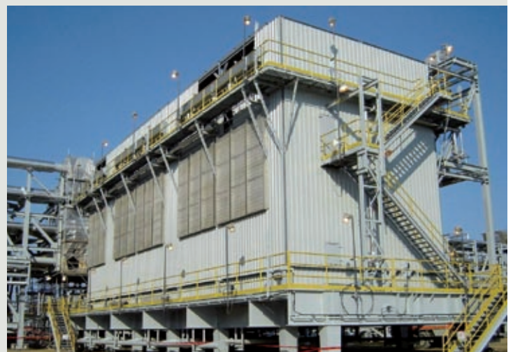
Air cooler installed in a gas complex in Sakhaline, Russia
