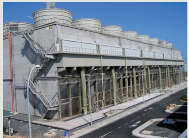
Plume-abated cooling towers of Plana del Vent, Spain
