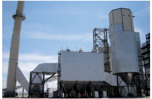
Fabric filter for a power plant in the Rockies, USA
