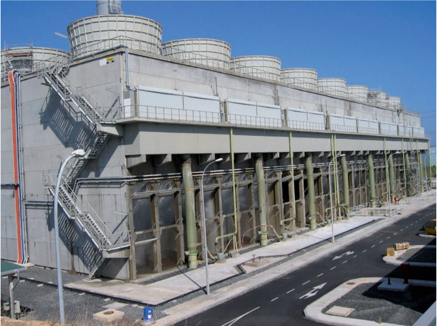
Plume-abated cooling towers installed by Hamon in Spain
