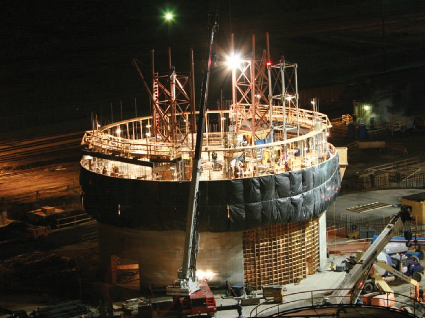
Upper platform of sliding scaffolding used in the construction of a chimney
