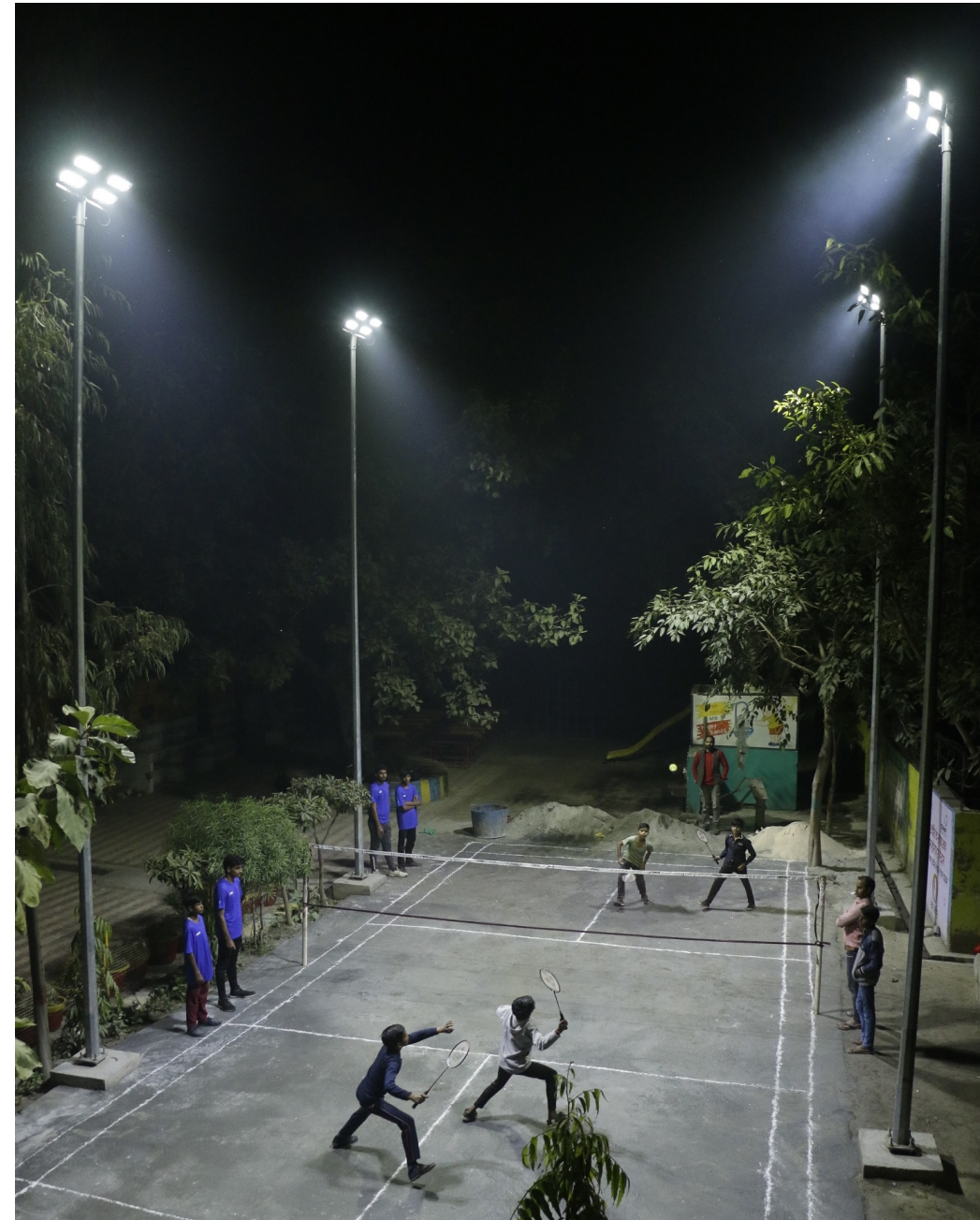
Solar-powered flood lights – Govt. Middle School – Rasoolpur Dasna – Dadri Block – UP – India
