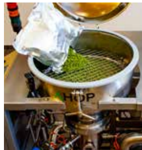
Agidens - Ahop dry-hopping installation
