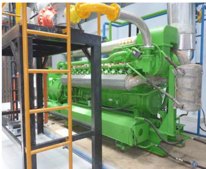
SIPEF - Biogas generator
