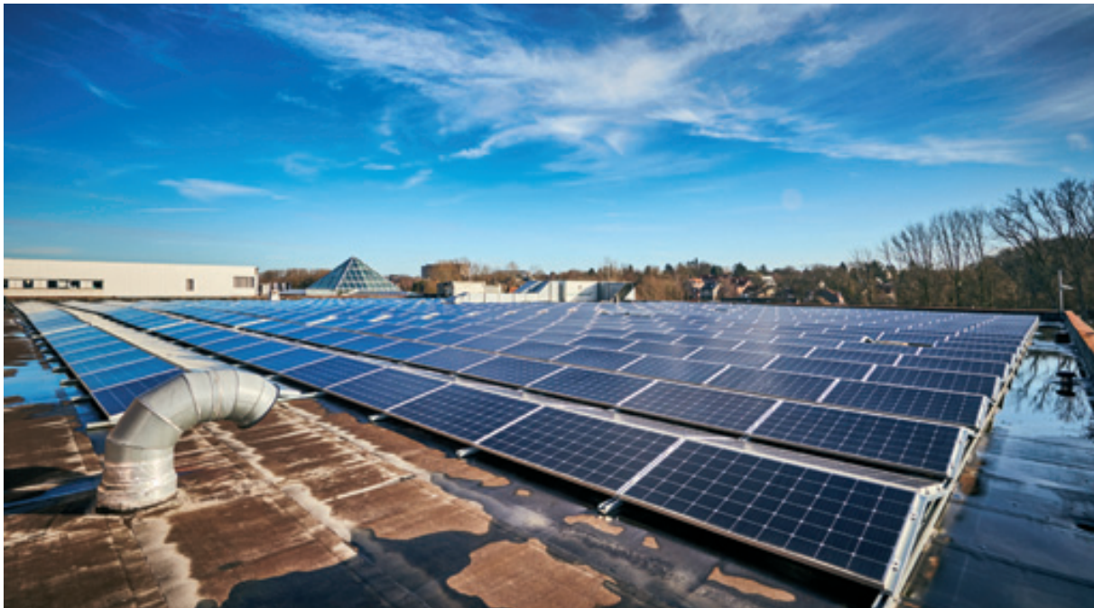
Solar panels on the roof of Woluwe Shopping
