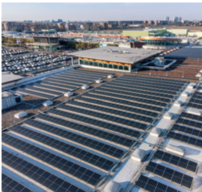
Roof solar panels at Fiordaliso
