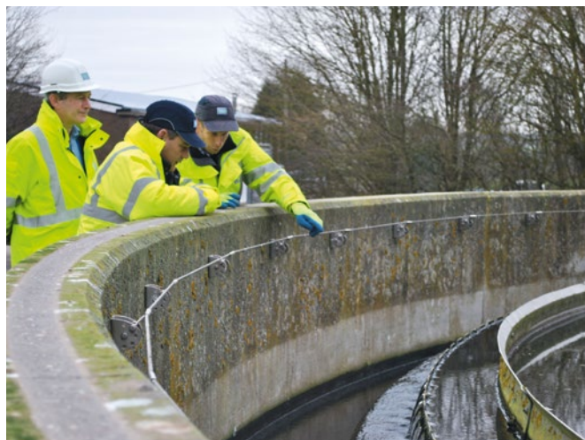
Inspecting the condition of our waste water assets at Packington treatment works.
