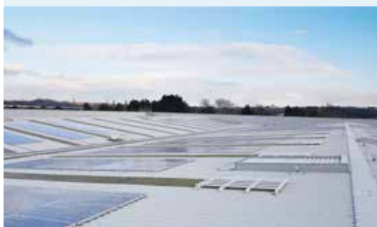
Solar panels at B&Q Poole
