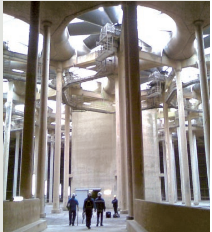
Inside view of a mechanical draft cooling tower built for a nuclear power plant in France
