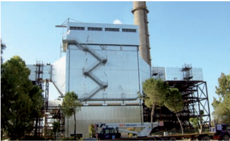
ESP built in a petrochemical plant in Italy
