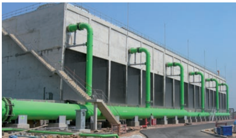
Mechanical draft cooling systems installed in Thailand
