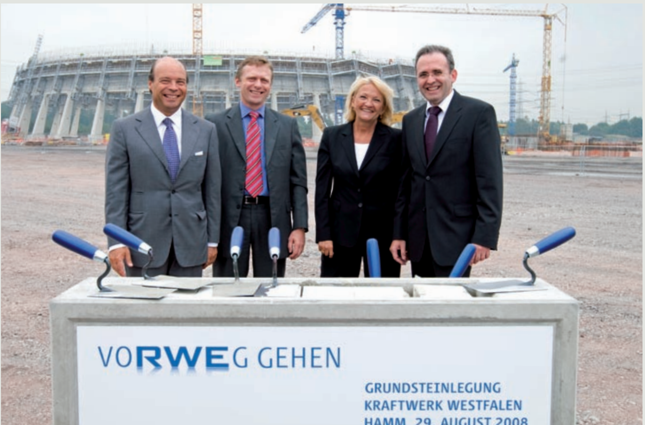
Beginning of the construction works for a natural-draft cooling tower in Germany (picture: André Laaks, RWE AG)
