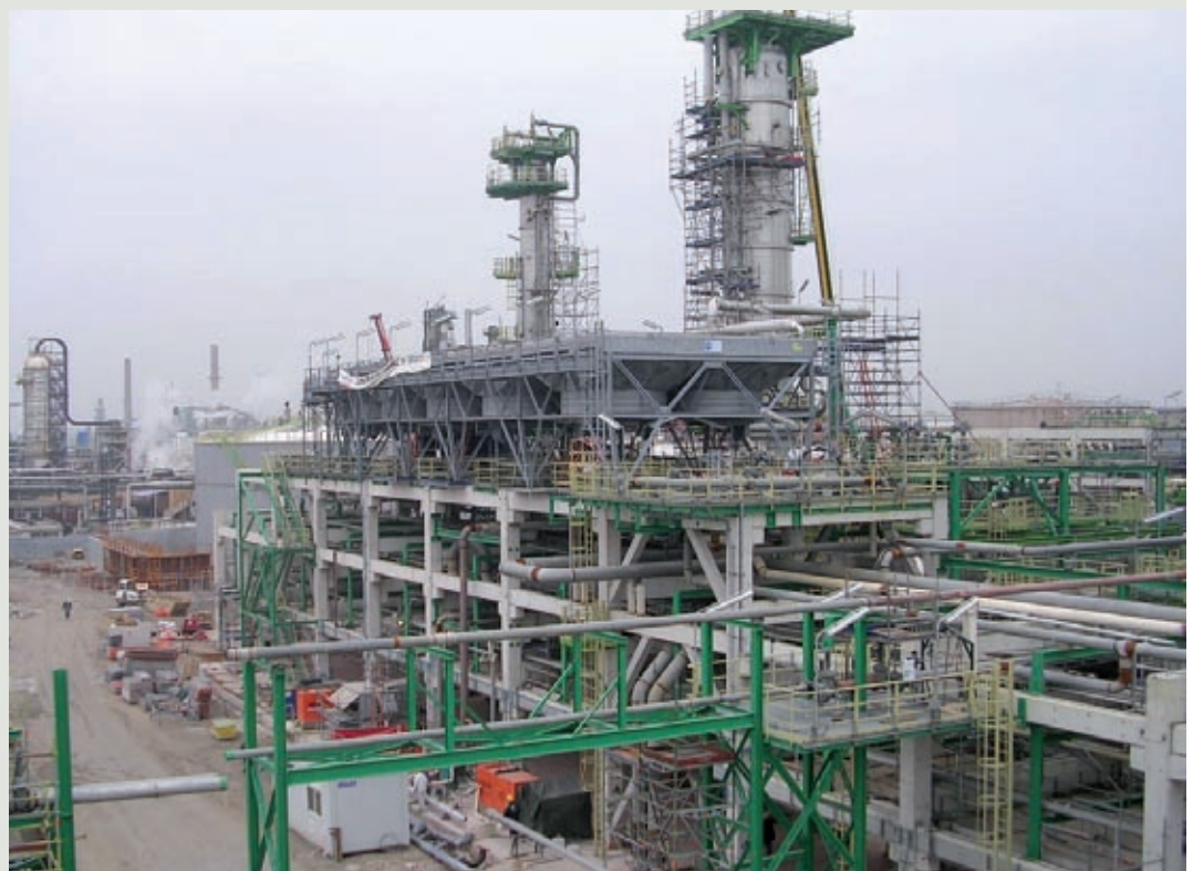
General view of a refinery and its air coolers
