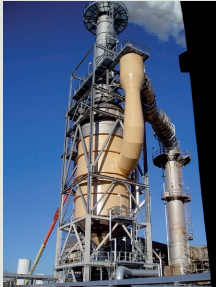
Wet gas scrubber built in USA
