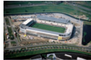
The new ADO stadium on the Prins Clausplein in The Hague, at the junction of the A4 and A12 motorways, has space for 15 000 visitors. The stadium was built between January 2006 and May 2007.
